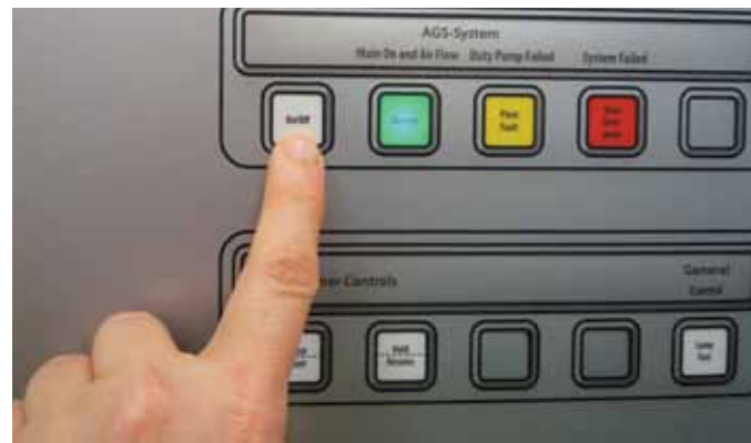
In most modern operating rooms the AGSS control is on the theatre control panel
